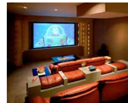
Custom Installation by Ambiance Systems, Clifton Park, NY
